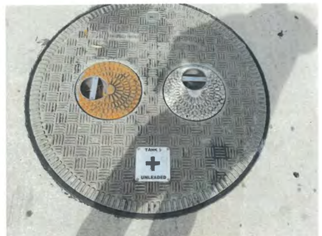
Tank 3 Unleaded Fill Sump
