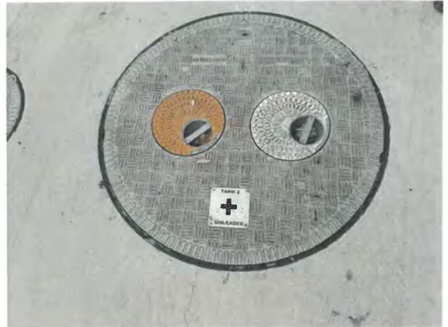
Tank 2 Unleaded Fill Sump
